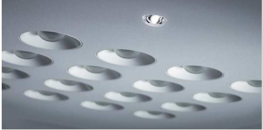
Integrated emergency lighting in R7 – webref. SKI001A3
