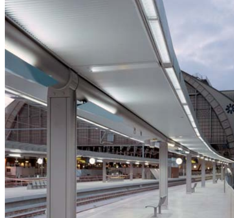
Central Station, Antwerp – Belgium (LON® system) – webref. SKX030C1
