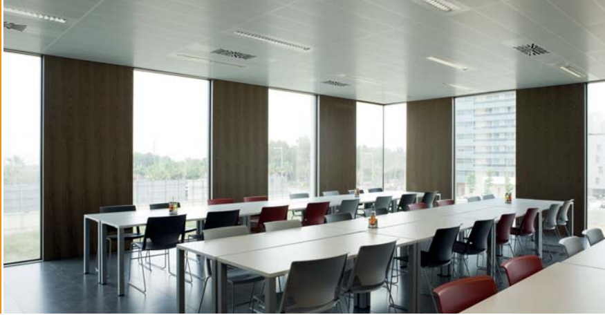
BLOOD AND TISSUE BANK OF CATALONIA - SPAIN - integration of emergency lighting into lighting luminaires - webref. SUX007G1
