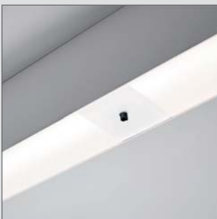
Daylight-dependent light control (ELS)
